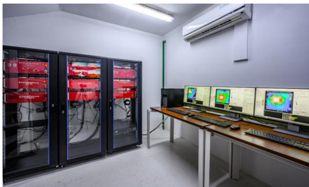
Fig. 2. control room underground with all receivers and control units.
